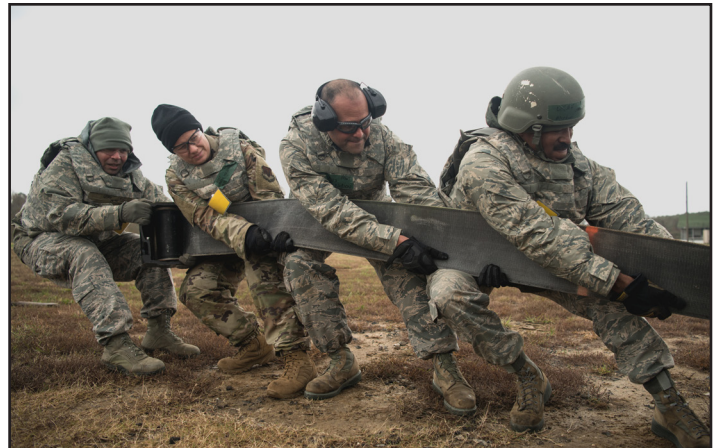
Virginia National Guard Airmen assigned to the 203rd Rapid Engineer Deployable Heavy Operational Repair Squadron set up a mobile aircraft arresting cable Nov. 16, 2019, during a four-day field training exercise at the State Military Reservation in Virginia Beach, Virginia.
